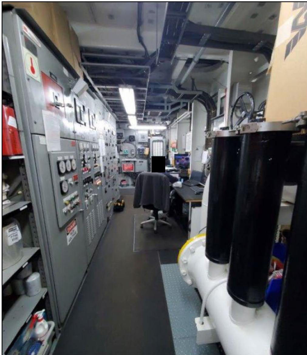
Figure 35: SEACOR POWER Engine Control Room (Exhibit 202)
