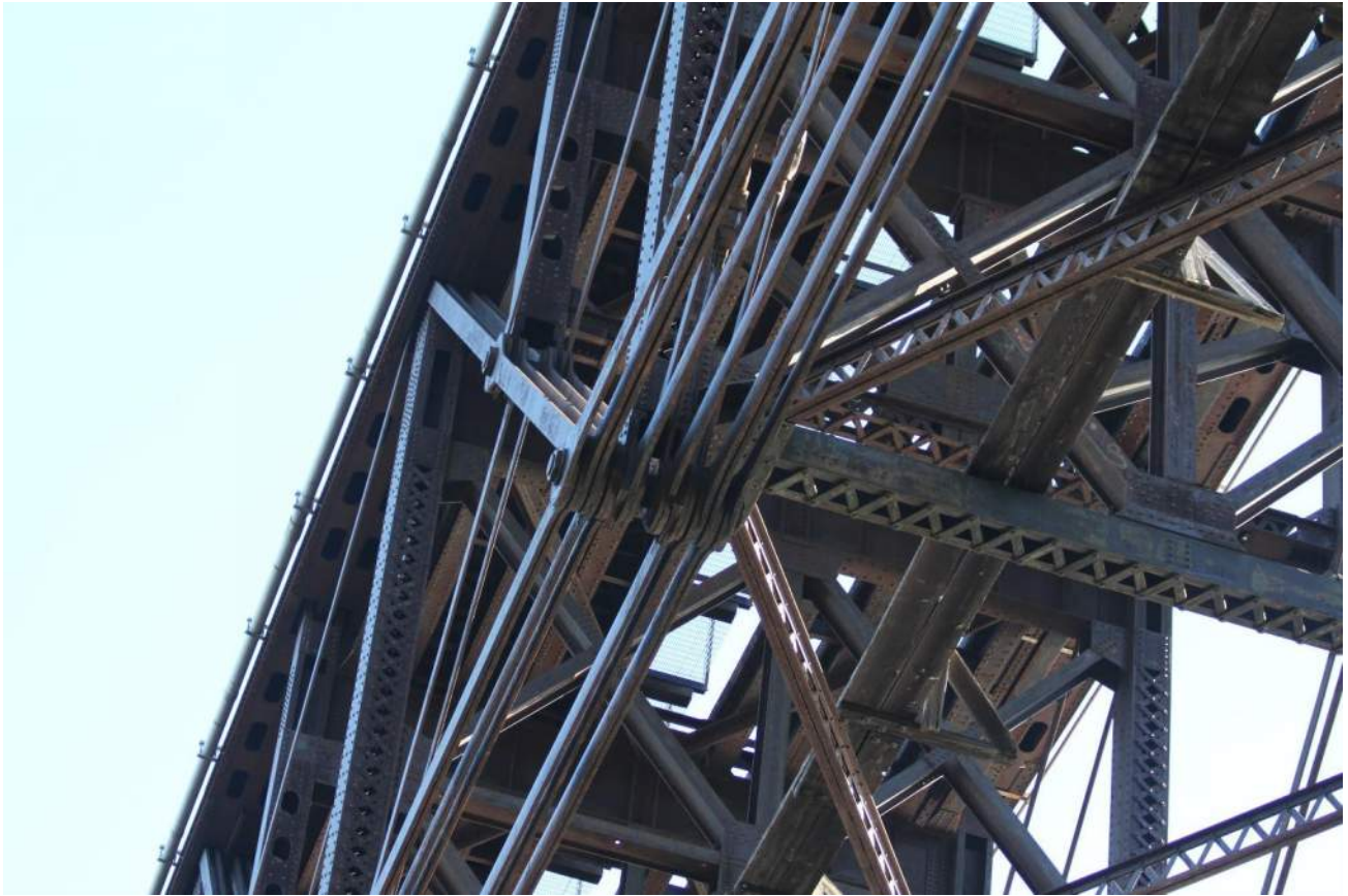
Exhibit B9: Typical pin and eyebolt connection, north face looking south east
