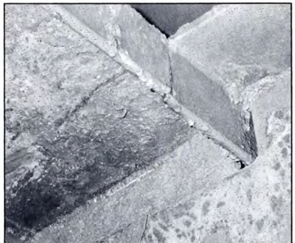
Corrosion in structural member of tanker ballast tank Photo by LCDR Steve Ciccalone
