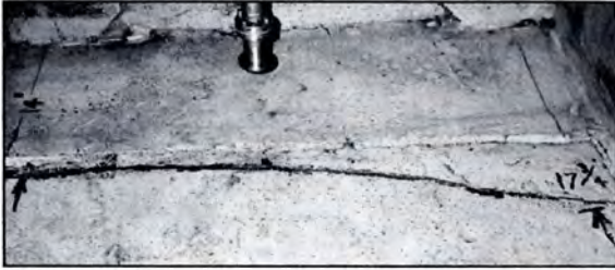
Portion of 20-foot long fracture in ballast tank bottom of TAPS tanker. Crack was 14 inches from an oil tank.
