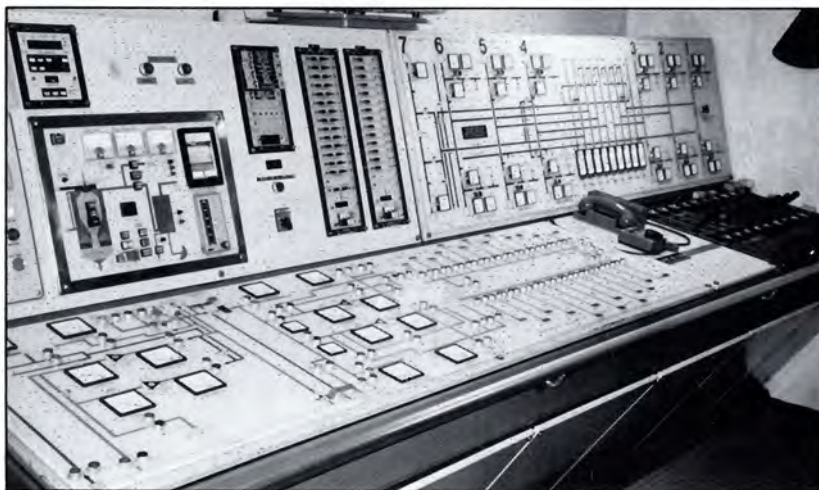
One-man main cargo control station aboard modern tankship.
