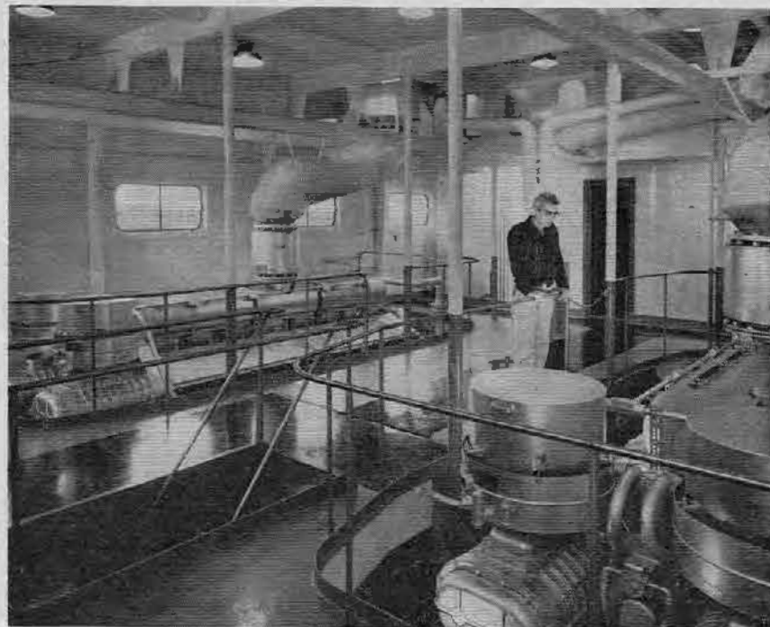
Well lighted and airy, this engine room is a model of compact towboat design.
