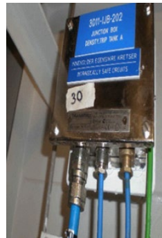
Improper Cable Gland Installation/Modification
