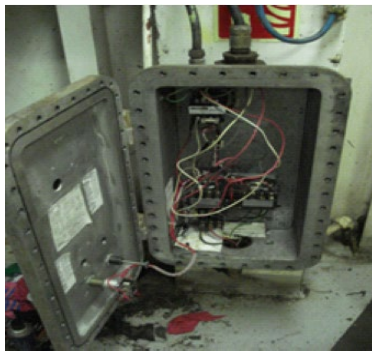
Improperly Modified & Maintained Certified Safe Junction Box
