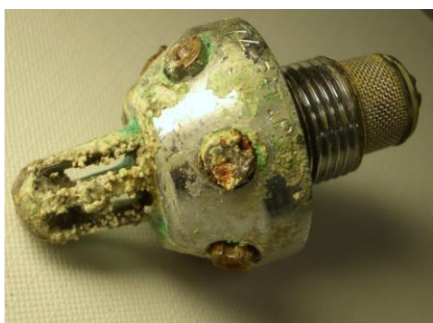
Picture 2 Severe contamination
