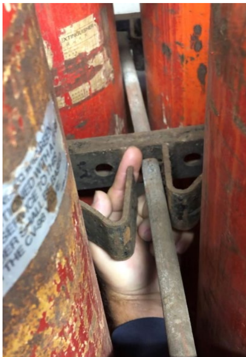
Failed Cylinder Bottle Brackets
