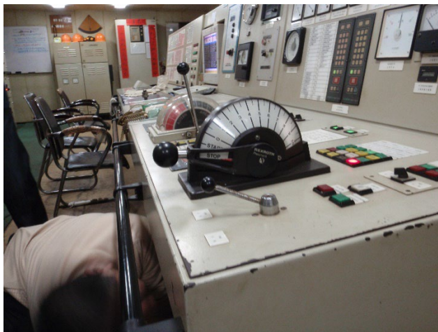
Photo shows Engine Order Telegraph control head.
