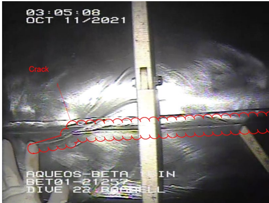
Figure 13 Still image from diver survey showing cleaned and buffed longitudinal crack (provided by Amplify)
