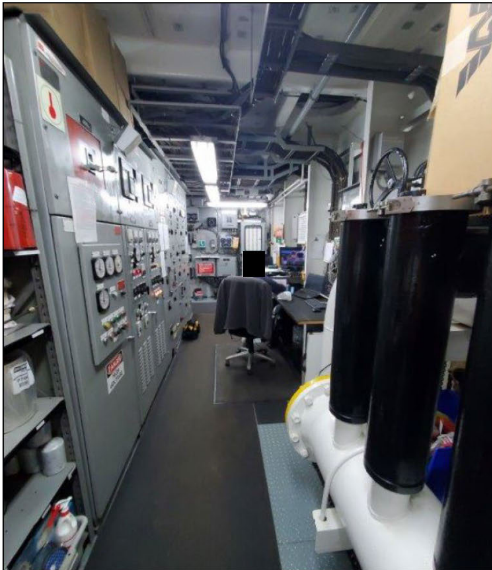
Figure 35: SEACOR POWER Engine Control Room (Exhibit 202)
