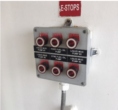
Figure 2. Aft deck emergency shut off. Taken on October 20, 2023.
