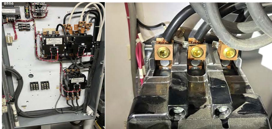
Figure 3. Inside of panel and high voltage conductor with fingerprints. Taken on October 14, 2023
