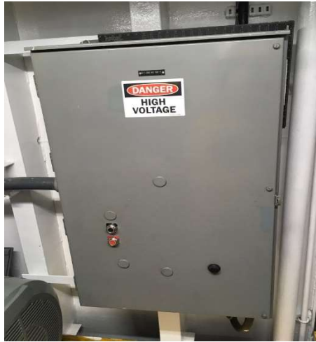
Figure 5. Mud Pump operation panel. Taken October 20, 2023
