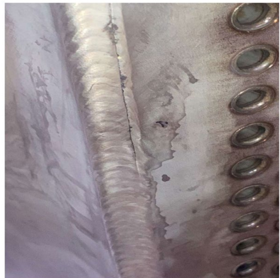
Close-up of cracked weld
