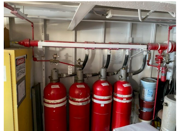
Figure 1. Fixed Halon fire extinguishing system.
