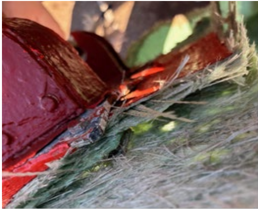
Figure 3: Close up of delamination at the hook attachment point.
