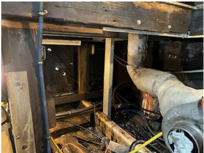
Figure 1 – Main Engine Dry Exhaust
