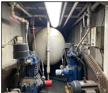
Fig 1 - Compressors & Air Receiver
