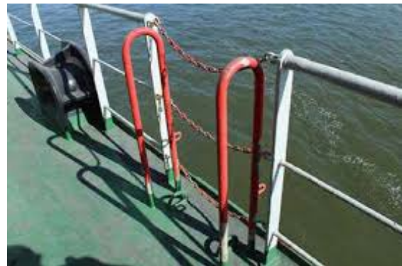
Figure 3: Handholds rigidly secured to the vessel structure at their base.
