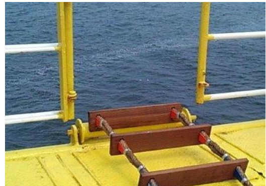
Figure 1: Handholds that terminate above the vessel structure.
