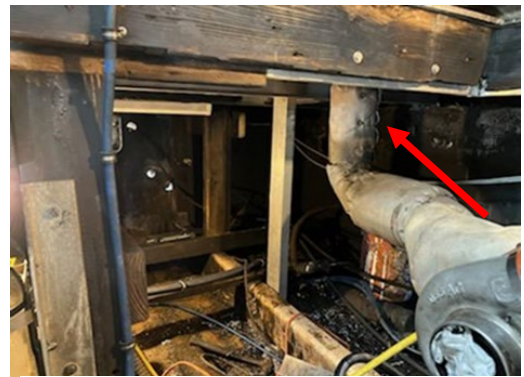
Dry exhaust passing through wood/FRP deck
