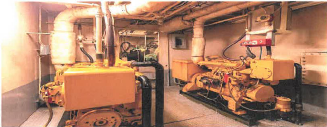
Figure 26: EMMY ROSE generator set, looking forward. Image Courtesy of Atlantic Brokerage.
