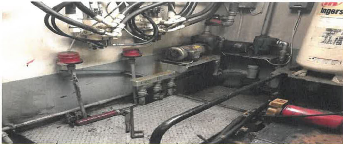
Figure 30: EMMY ROSE bilge manifold system. Image courtesy of Marine Safety Consultants.
