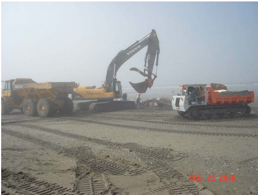
Photograph taken August 23rd, of the removal of the wrecked FV ILA.
