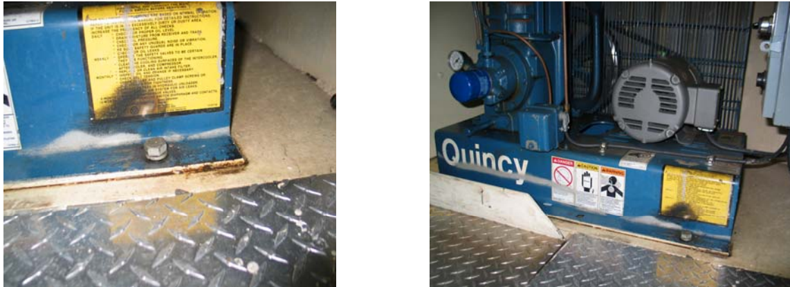
Figure 44. One company intends to reduce noise and vibration by replacing these current compressor mounts with sound-deadening ones.
