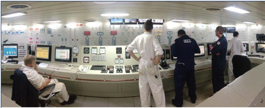
The engine control room on a modern cruise ship. Photo credit: LCDR Eric Allen, USCG
