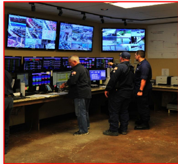
Coast Guard personnel observing the security and safety control systems at a marine terminal. USCG photo
