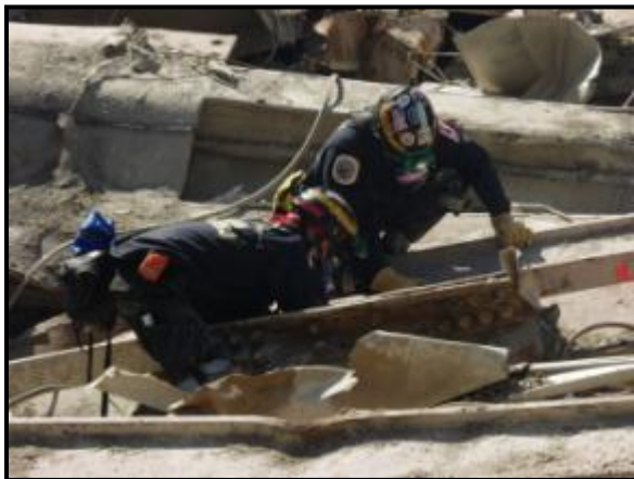
(09/27/01) California Task Force-3 personnel work on cutting steel and clearing rubble at the collapsed World Trade Center, New York City. (Photo: Michael Rieger)
