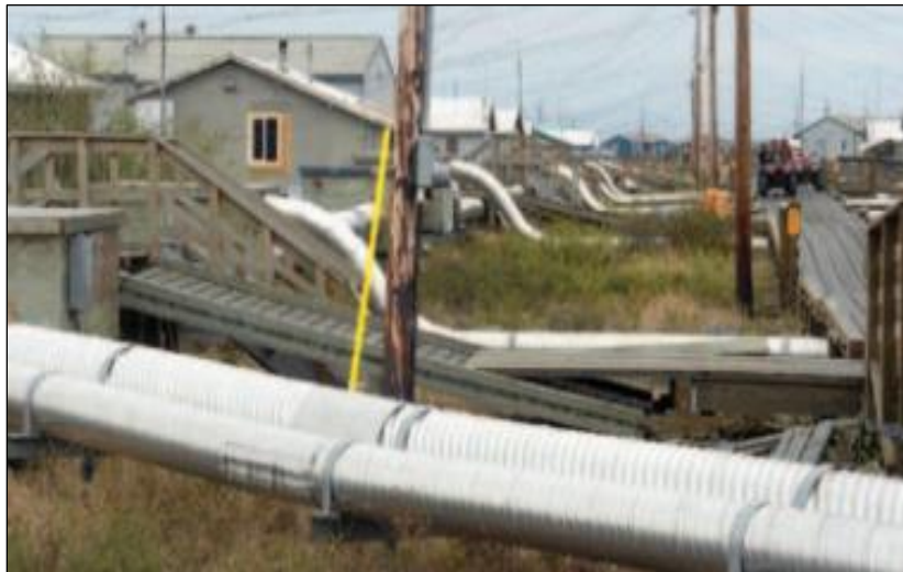
Figure 2. Exposed Water Pipes Can Be Seen Throughout the Village
