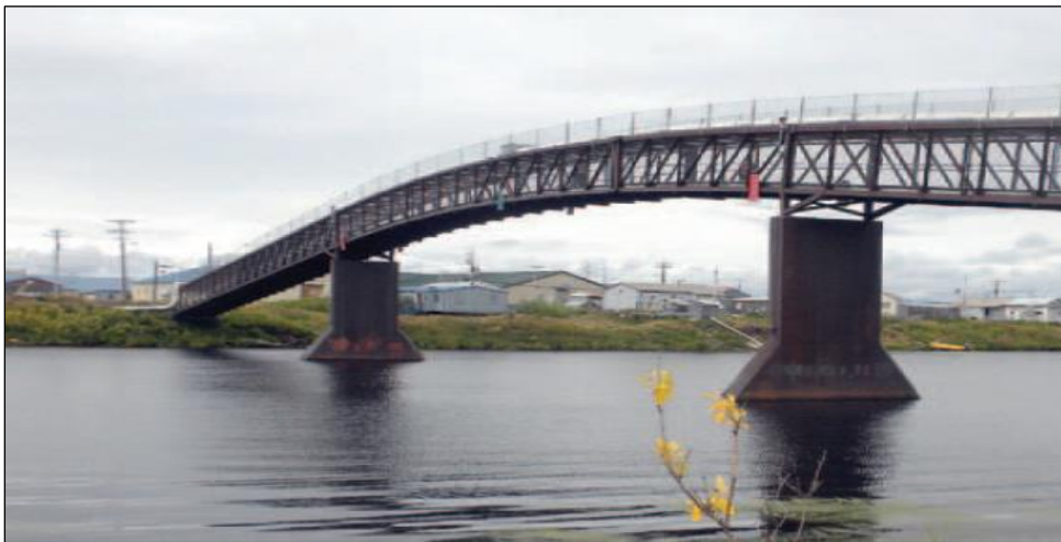
Figure 7. Rainbow Bridge is Gradually Sinking into the Selawik River
