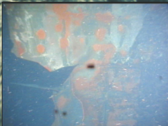
This photo shows structural damage from the explosion, which is indicated by the way the plate is torn and bent outward.
