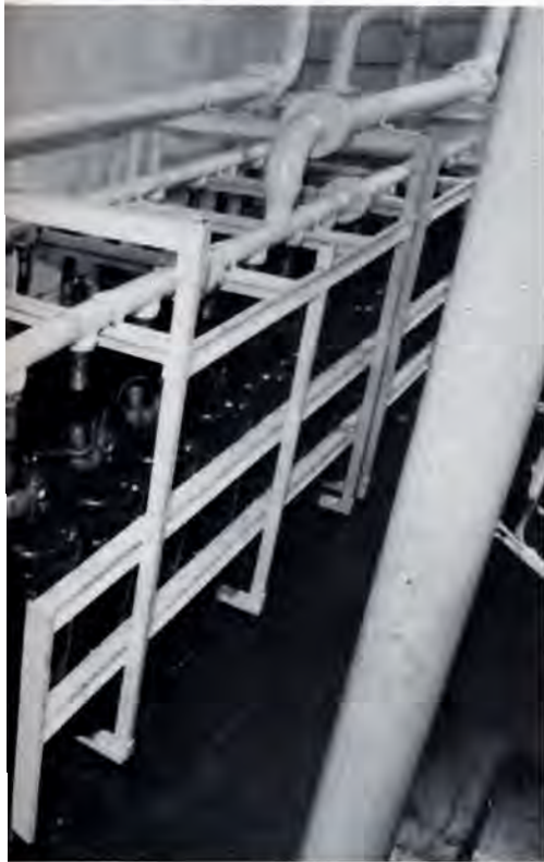
A typical halon installation
