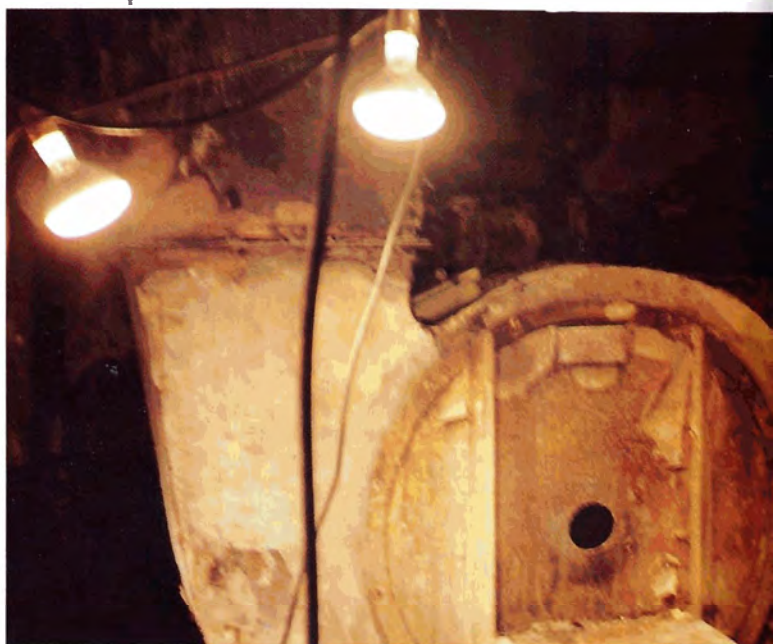
Motor and fan impeller removed.
