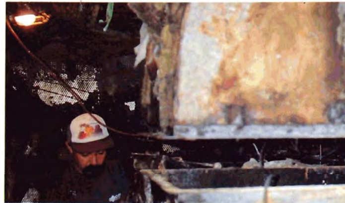
Canvas ducting burnt away.
