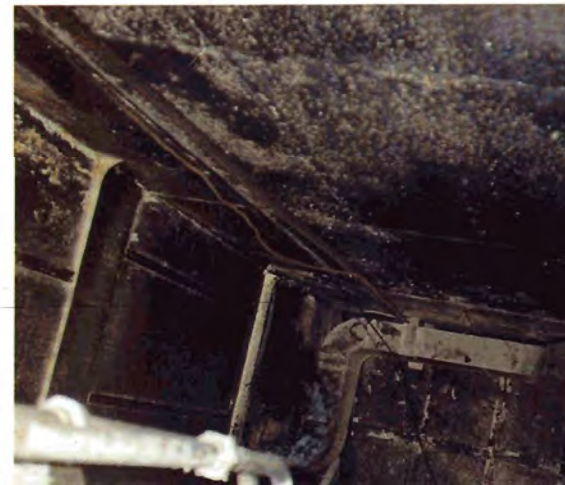
Supply trunk looking from base of mast down into fan room #4.
