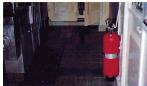
Fire extinguisher adjacent to braising pans.
