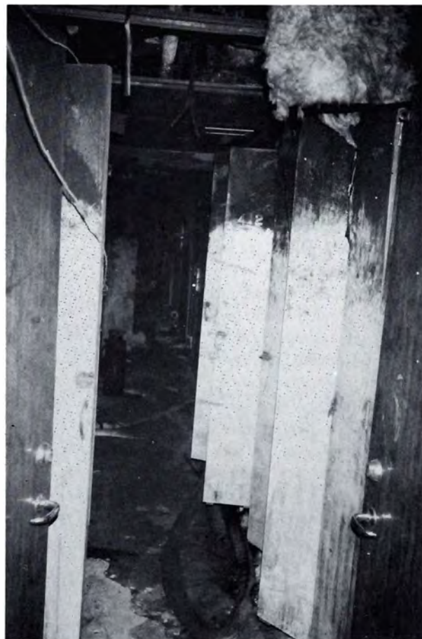
Burned finishes and soot along the top of this corridor show what can occur during a fire at sea. The vessel had fire detectors, but no automatic sprinkler system.
