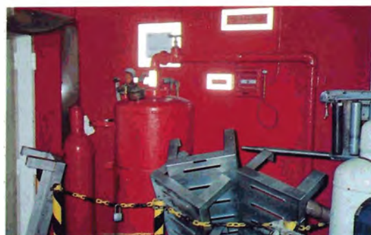
Foam fire-fighting system for crew galley lower duct.
