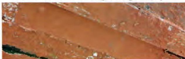
Bulging plank indicates break in smooth hull lines.
