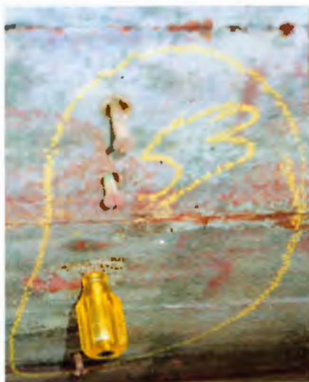
Awl penetration beyond fastening depth indicates rotted frames and no holding power for screws.
