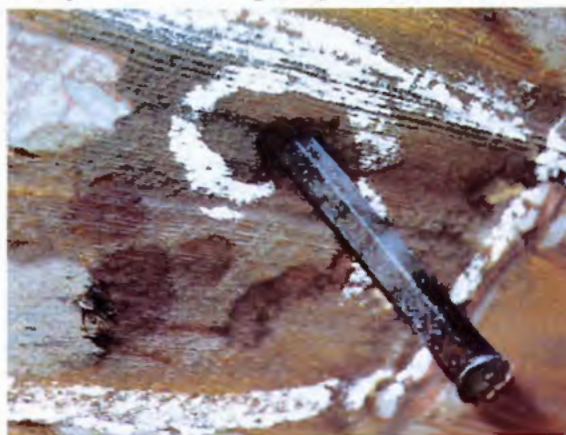
Drift (used to sound boat nail fastening) penetration beyond plank thickness indicates soft wood structure.
