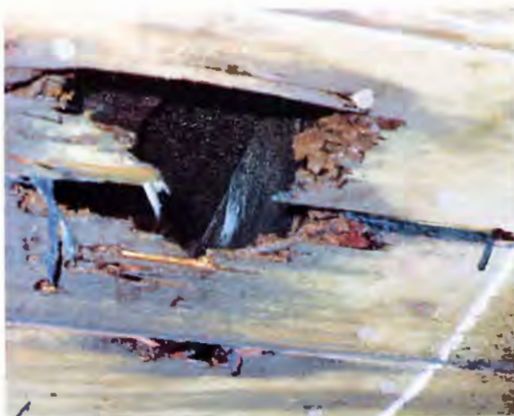
Planking rotted from inside out, found by outside sounding.
