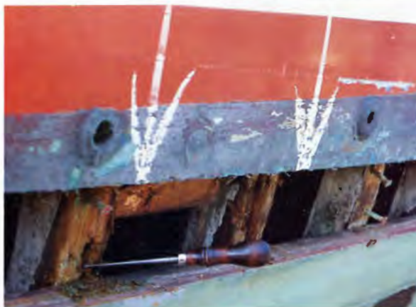
Rotted framing behind plank pulled for inspection.
