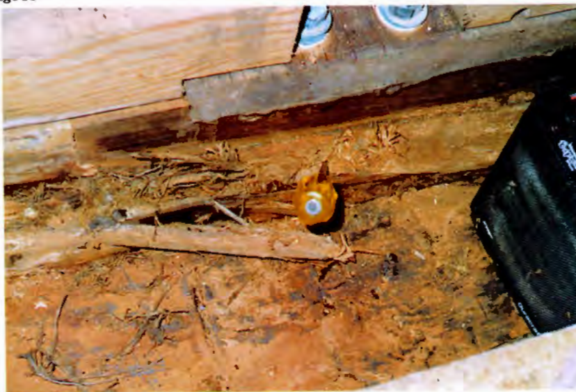
Floor timber rotted due to fresh water accumulation and lack of drainage.
