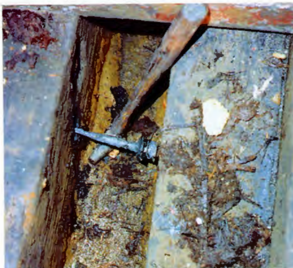
Deteriorated floor timber to frame fastening.
