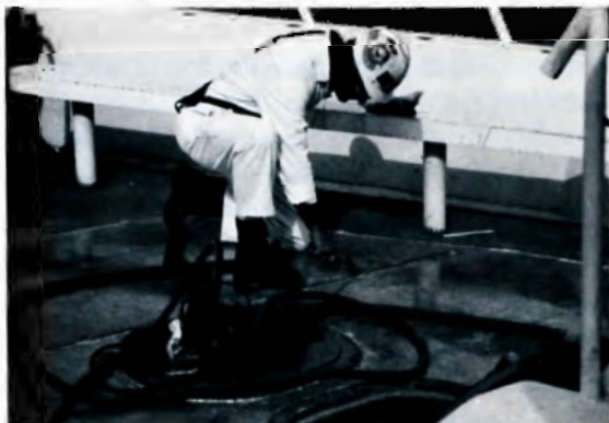
Coast Guard inspector examines repairs to foredeck.
