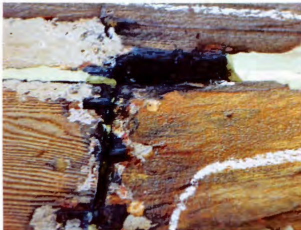
Open seam and over-fastened butt caulked with water-setting epoxy.
