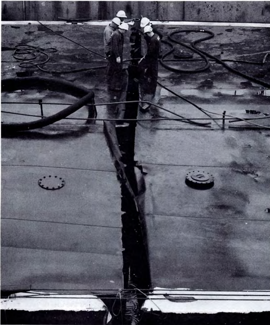
Inspectors survey damage to the deck of a tank barge which resulted from structural damage.
