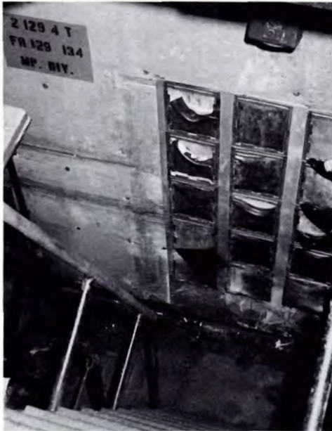
Intense heat damage to the main escape route from the boilerroom.
