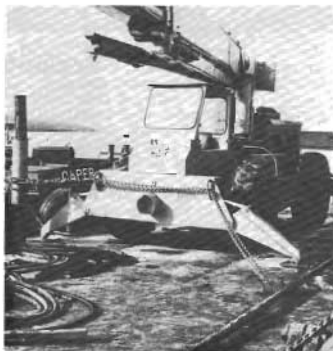
The crane operator was unfamiliar with the type of boom used in the Grove RT-58 crane, the telescoped section of which is barely visible at the top of this photograph.
