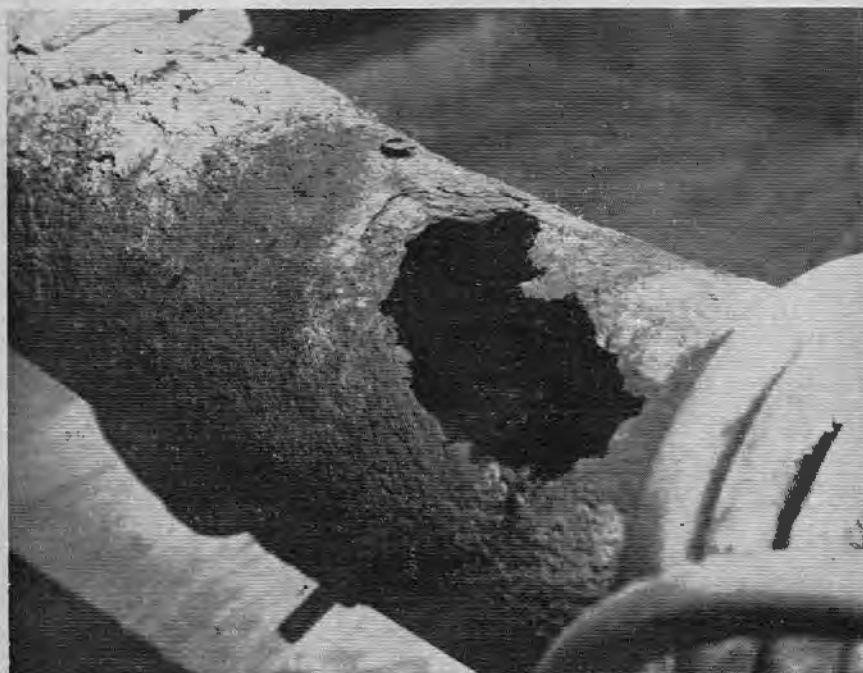
Figure 1.—Section of exhaust line showing hole and coil of tubing which hid it from view.
