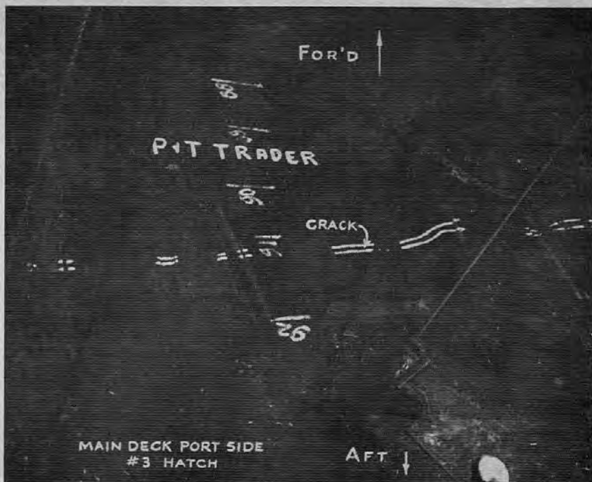
Figure 1. Looking forward on port side main deck of SS P & T Trader showing crack and emergency welding repairs.
